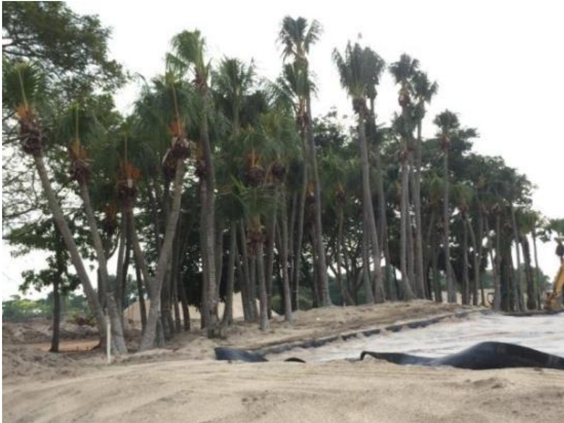
Above: A special nursery space was set aside on the project site to facilitate the relocation of 268 palm trees
