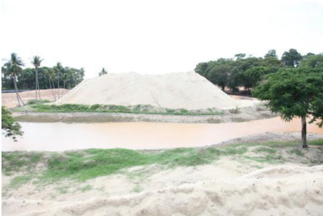
Above: Valuable greens mix and fairway sand were harvested and stockpiled to be re-used once the new golf holes were ready for shaping.
