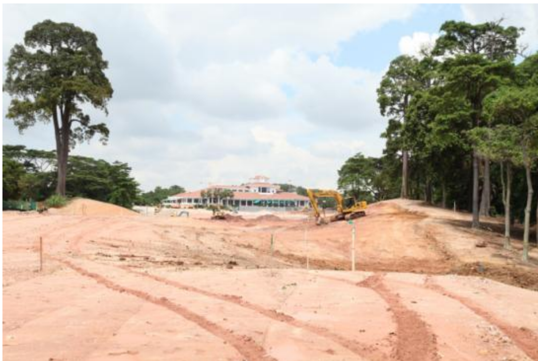
Above: The old Tanjong course was home to a few large grooves of mature trees. These areas were safeguarded in the design and routing of the New Tanjong Course.
